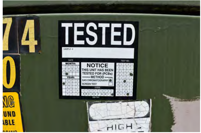
32. Pad-mounted transformer eastern portion
