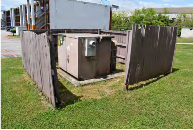
31. Pad-mounted transformer eastern portion
