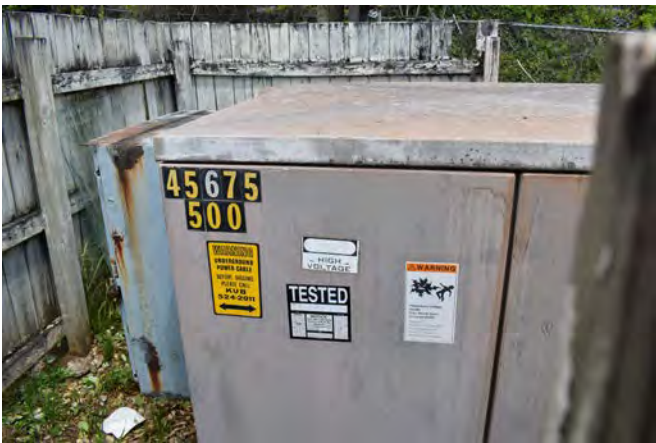
33. Pad-mounted transformer western portion
